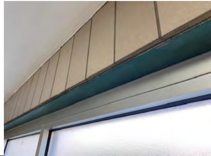
Exterior and Interior Building Throughout. Metal Lintels (Older) with LBP identified.
