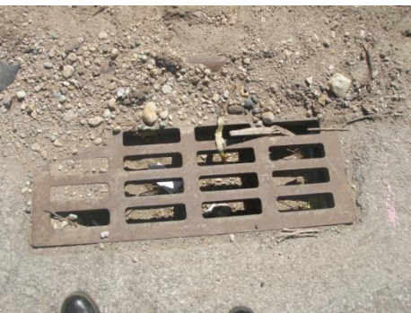
Inlet basket that is not being maintained.
