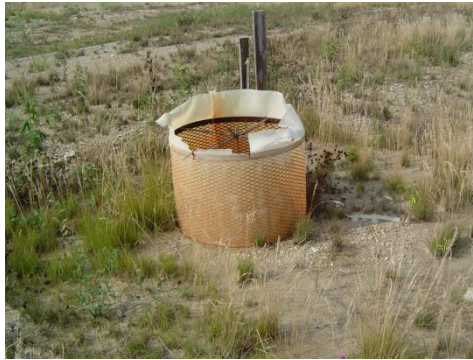
Protection around area inlet.
