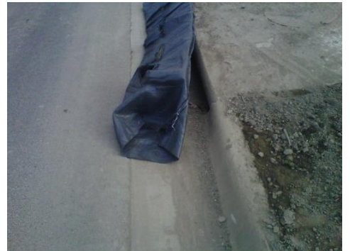
There should be no gaps on the upslope side That would allow sediment to enter the inlet.
