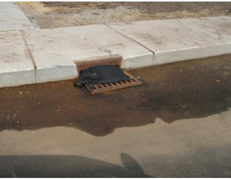
Inappropriate use of a rock sock over an Inlet.
