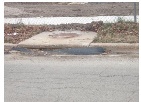
Rock sock inlet protection that is not being maintained.
