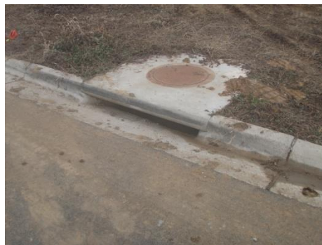
No inlet protection
