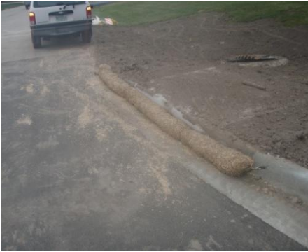
Straw wattle over inlet to keep sediment from laden storm water from entering the storm sewer.
